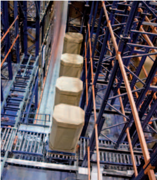
Hall with storage stacker
