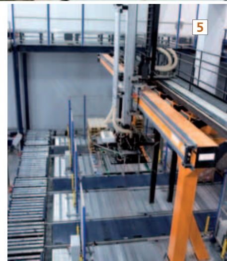
The automatic picking robot can prepare high turnover products in small multiples instead of larger lump groupings. The pallets are fed by the stacker cranes and automated warehouse containers.
